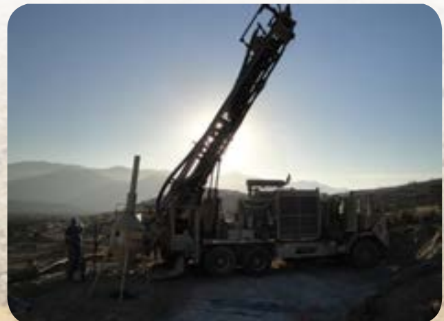
Drill rig at La Chulula, during the first RC drilling campaign in June-July 2012.
